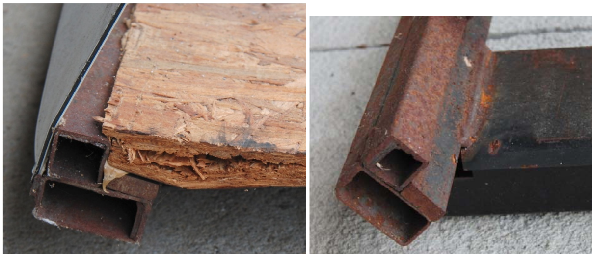
Figure 13: Mode of failure for wall to floor connections.
